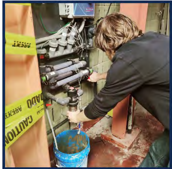
Top: Cooling 1's Chris Pelat checking corrosion coupon rack.
