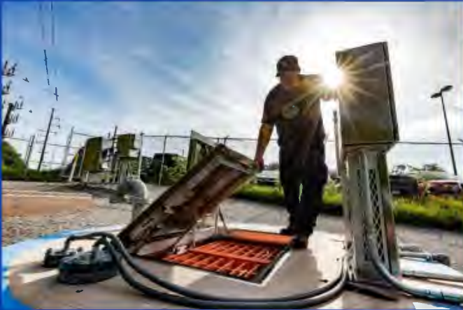
Figure 1 The Stormwater Harvesting wet well holds diverted stormwater for use in CUP. Photo taken by Arden Barnes on July 7, 2023.
