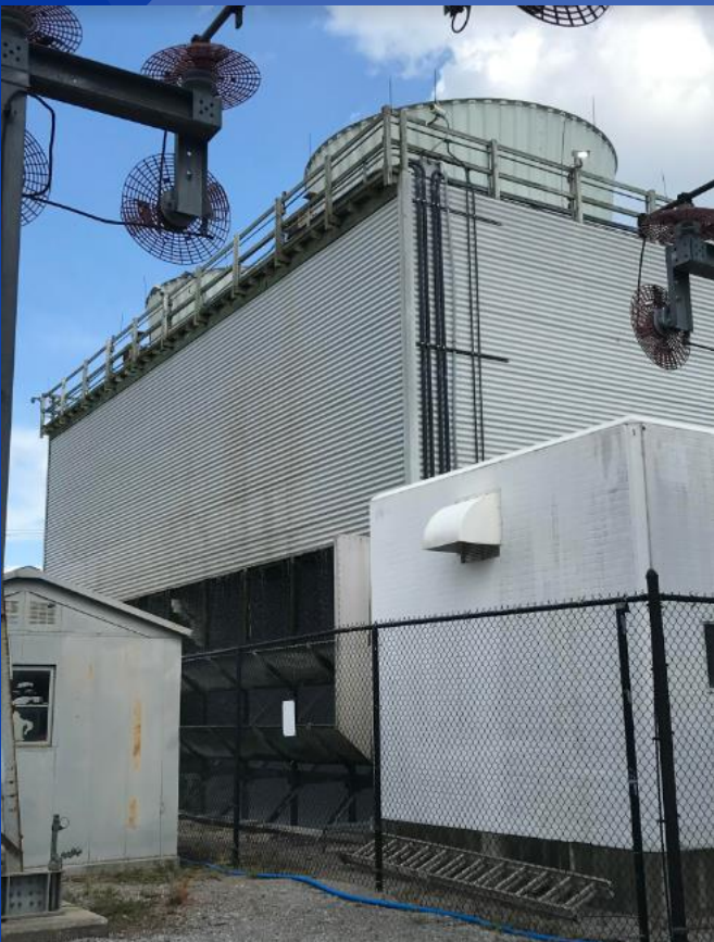
Figure 2 Cooling towers cool water for operations around campus. Photo taken by Jennifer Bukowski on August 29, 2023.
