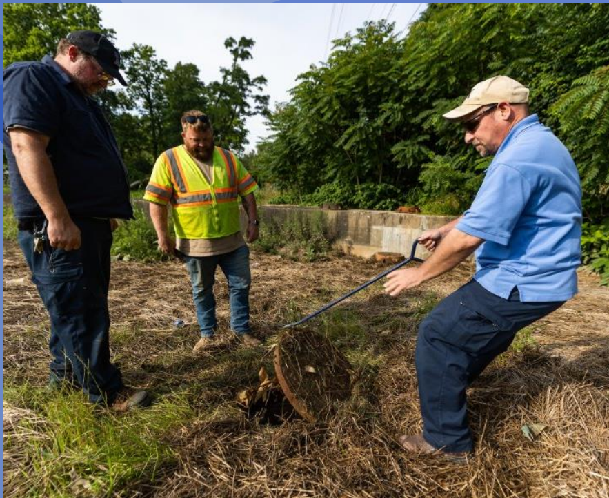
Figure 6 Regular cleaning of the system helps maintain its integrity and improve performance.
