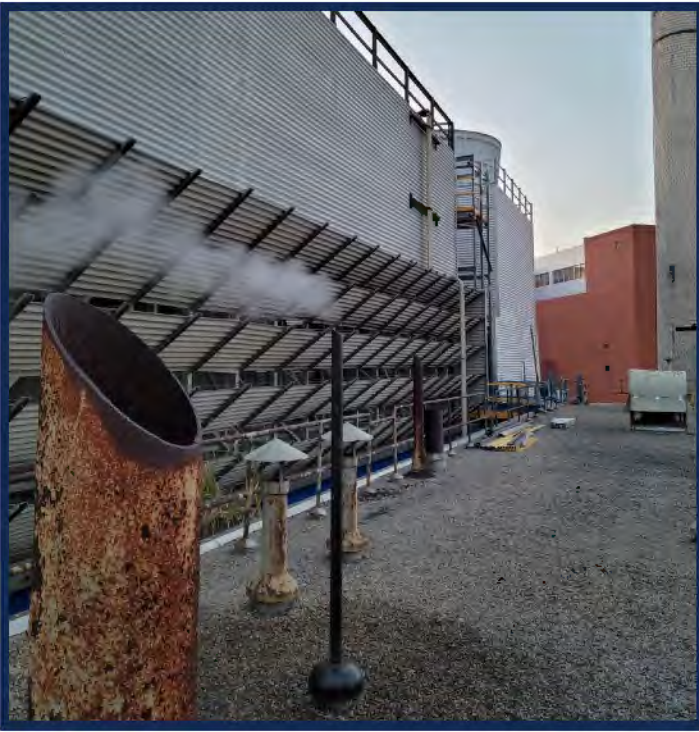
Top Left: The new and improved vent for the old DA tank at the Med Center plant. Right: David Derenge clearing the automatic blowdown at Cooling 1.
