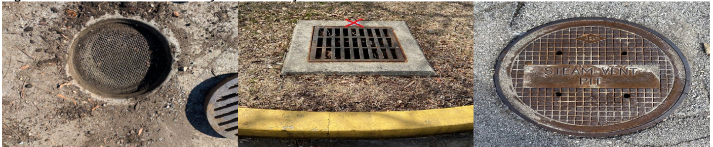
Figure 2: Photos of different utility vents. Utility vents should not be marked.
