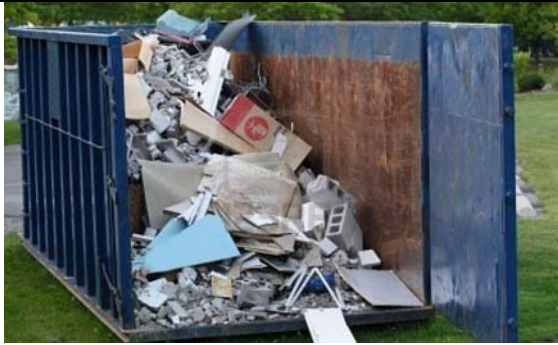
Construction waste and materials handling is part of any Stormwater Pollution Prevention Plan (SWPPP).
