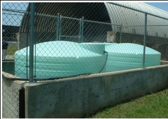
Secondary containment is used to protect the area in the event of a spill.
